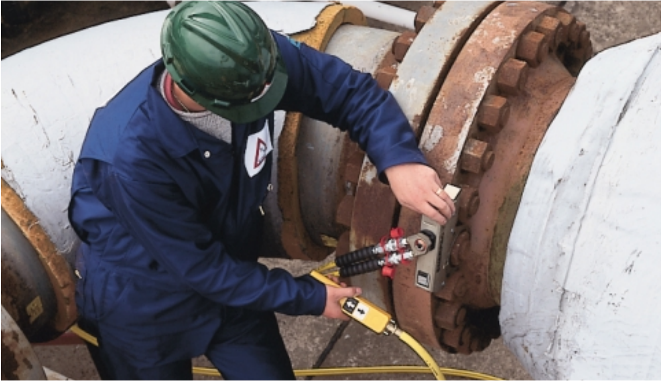
Using a hydraulic torque wrench, the bolted joint can be tightened in a controlled way, with the correct bolt prestress in conformity with designer requirements.
